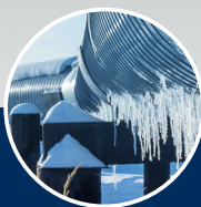
Moisture ingress & ice build up
